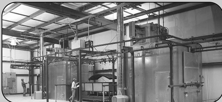
Our facility has large part PVC coating capability.
